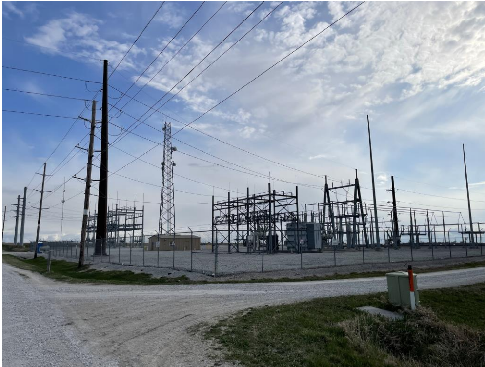
ITC Midwest's Ames substation north of Ames.
